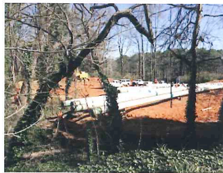
AGL staging area and site of the Gas Regulator Station, as seen from the back yards of adjacent homes. Courtesy of Lori Muskat
